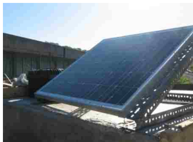
(a) Compact RIO and solar panel
